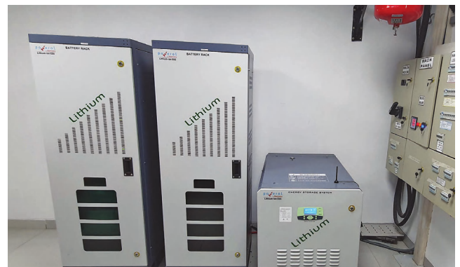
A lithium ion battery storage system at an ICICI Bank branch in Delhi.
